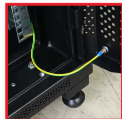
Grounding Connecting Between all Removable Part of Rack
